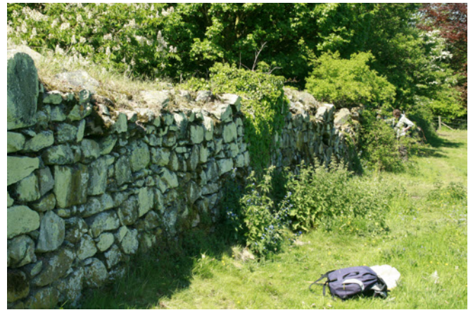
The northern section of the wall, east side, which receives full sunlight in the mornings.
